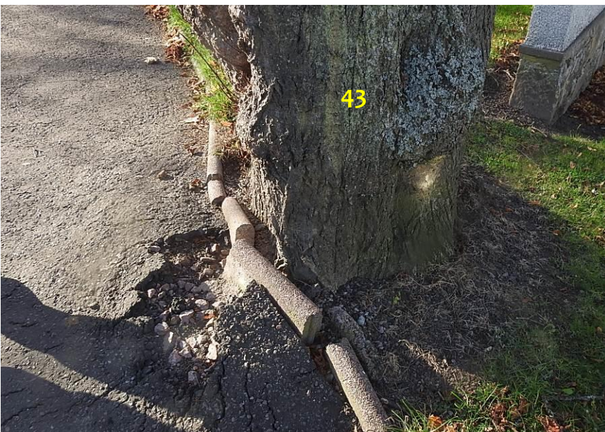
Photo 3: Lime 43, with root growth causing the pavement to be lifted. This pavement restricts the root growth of the tree. It is recommended that this tree is retained as any action will likely cause damage to the tree.
