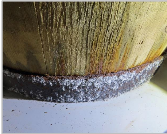
Salt efflorescence, corrosion and flaking of the iron
