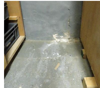
Damp/Salt plaster damage
