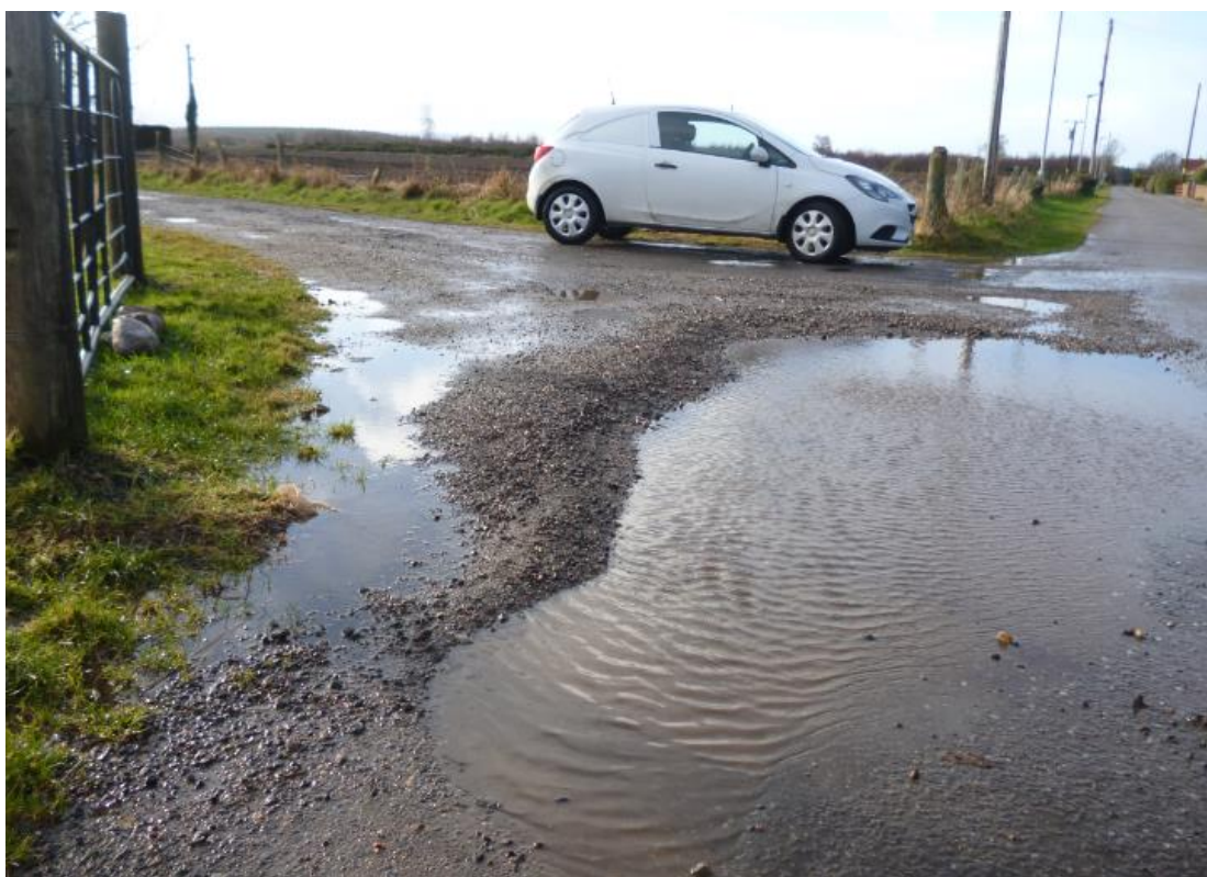
View into site access – note evidence of loose material/ water ponding
