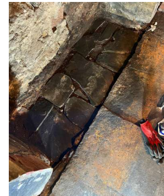
040 east living room original slate hearth bed exposed during 2022 part made up of roofing slates
