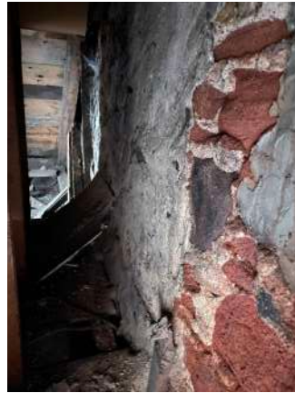
058 East bedroom - 1st floor void behind tank housing to gable wall
