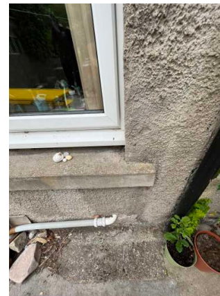
019 south elevation kitchen window concrete sill
