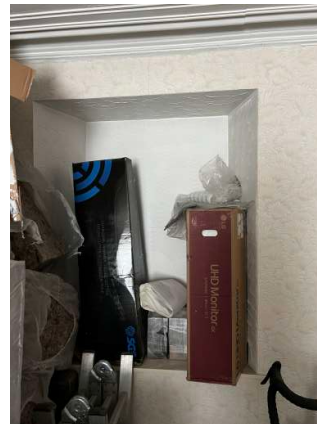
048 west living room rear/south wall original window blocked-up
