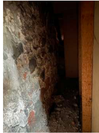
059 East bedroom - 1st floor void behind tank housing to gable wall
