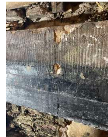
076 cracked fireplace lintel to east living room fireplace
