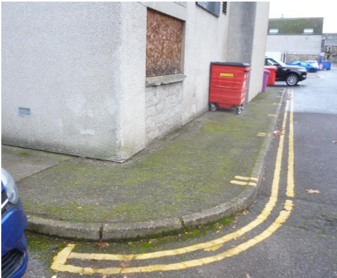
View (to east) of existing footway at proposed new takeaway entrance Batchen Lane
