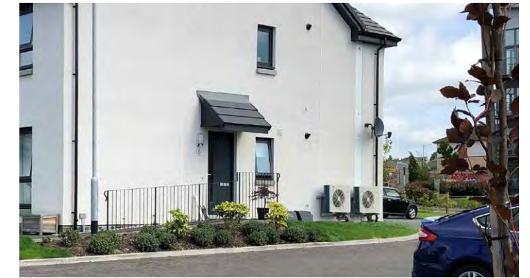
Air Source Heat Pumps
