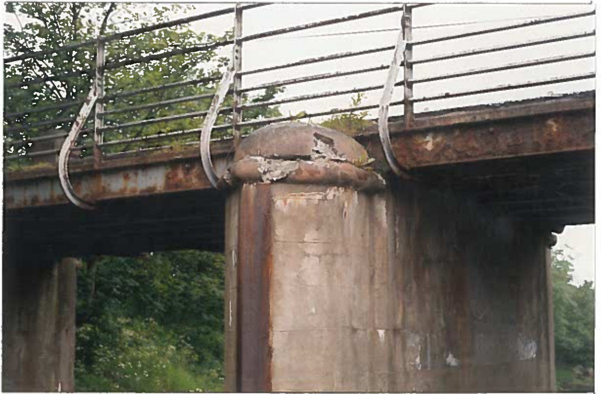
SPALLING OF CONCRETE ON PIER
