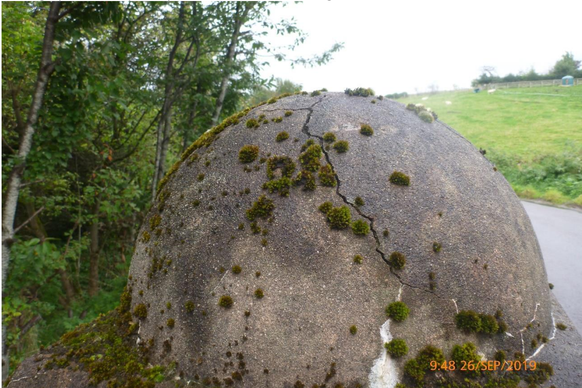
Photograph 34: Cracking of Wingwall parapet topping stone (North-East)
