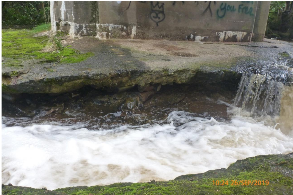
Photograph 24: Scour of bridge invert at centre span. Visible scour extending beneath invert on East side.
