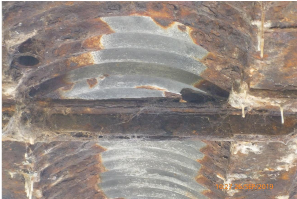
Photograph 16: Significant corrosion to parapet bracing member.
