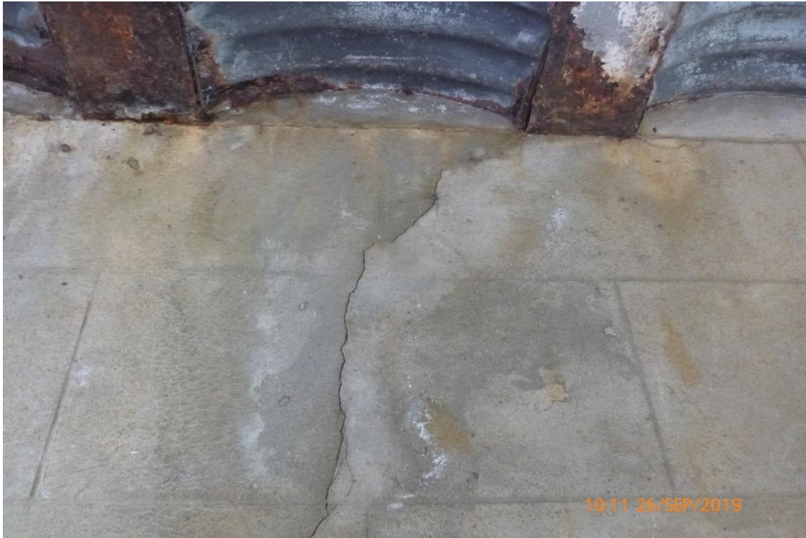
Photograph 18: Vertical Crack on West Abutment starting from beam (0.8mm).
