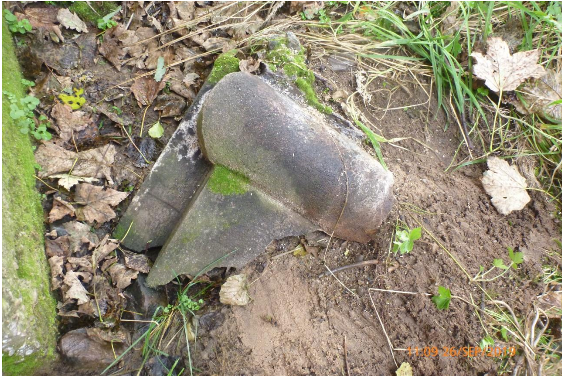
Photograph 28: Concrete breakout at East abutment / wingwall
