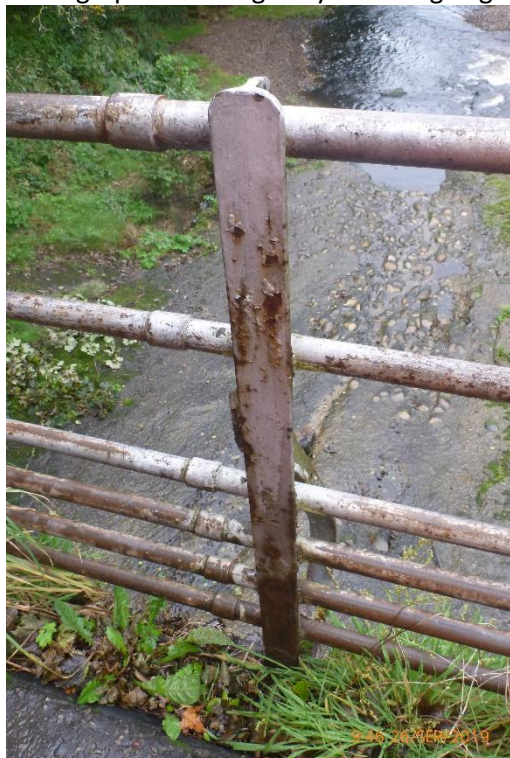
Photograph 8: Typical section of parapet corrosion.
