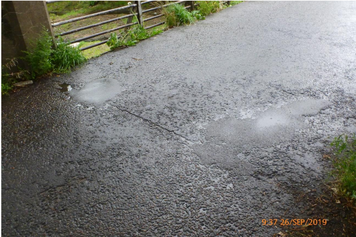
Photograph 7: Carriageway surfacing in good condition with minor patch repairs. No Joint visible.
