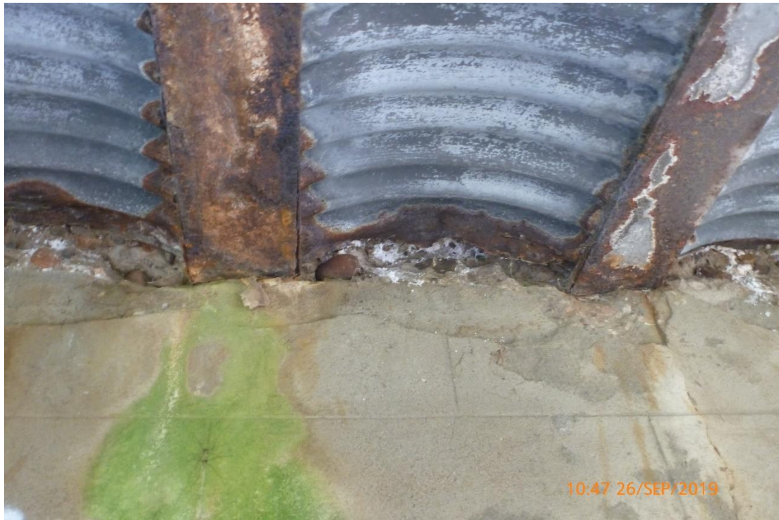
Photograph 20: Spalling of concrete between and under beams. Algae aggregate sizes visible
