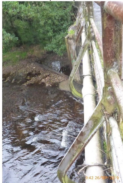
Photograph 9: View of pipeline passing through parapet bracing members on the South side.
