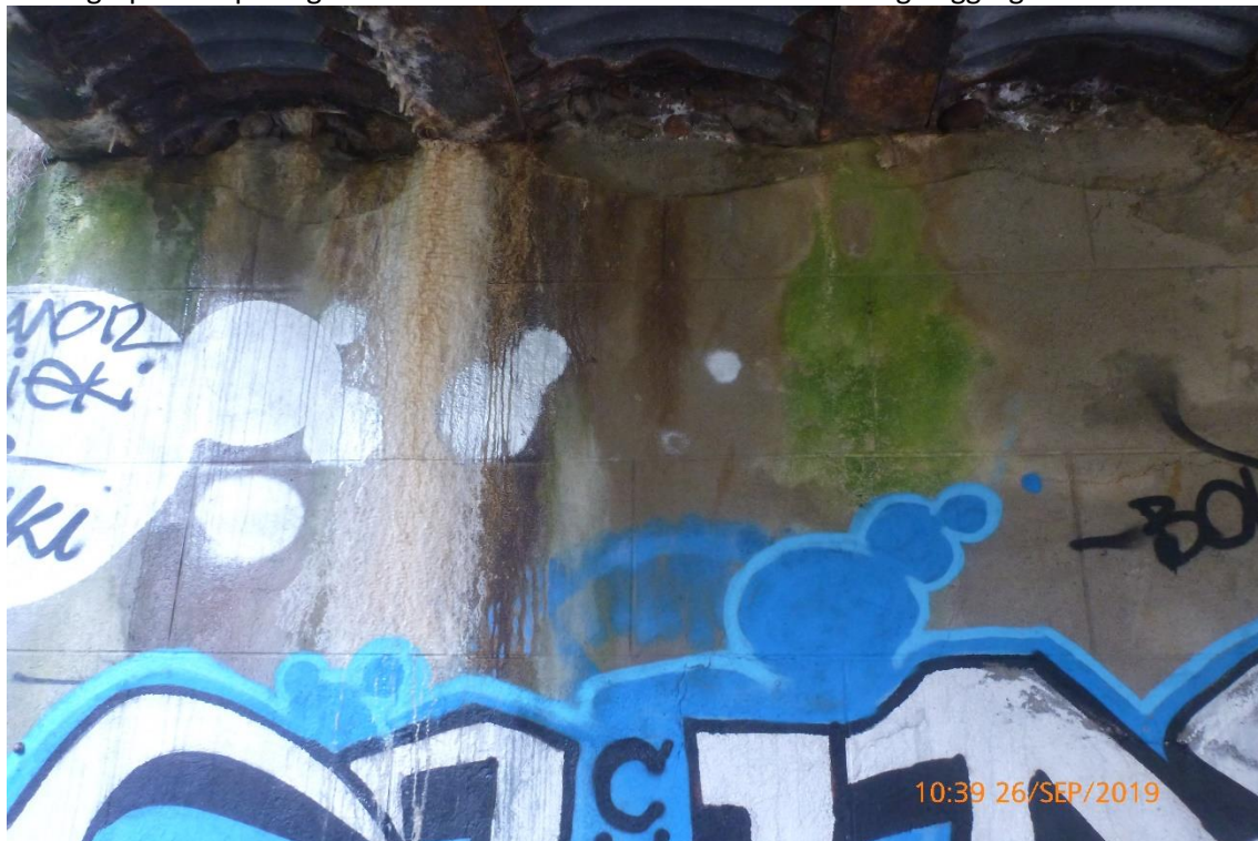
Photograph 21: Typical example of significant calcite build up on Abutment and algae staining.
