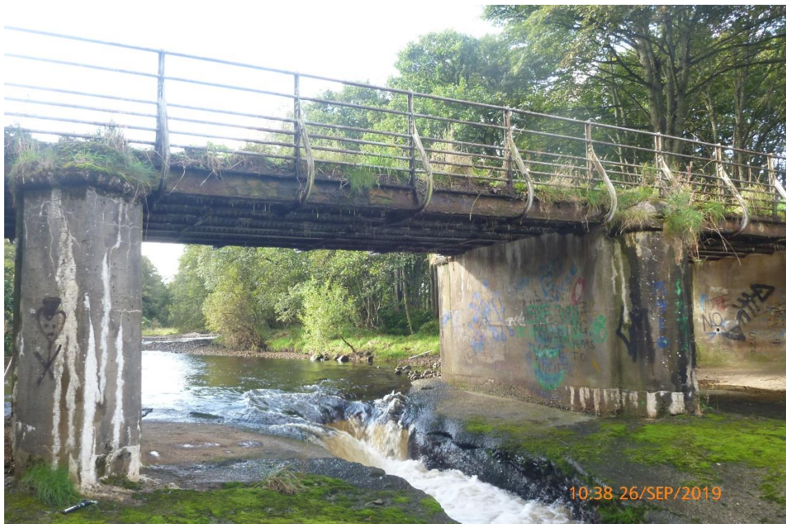
Photograph 25: General view looking South at centre span with invert scour.
