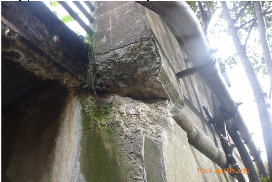
Photograph 27: Concrete breakout at East abutment / wingwall.
