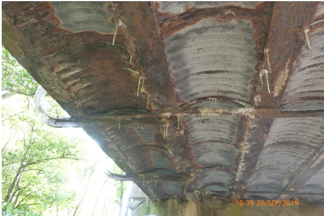
Photograph 10: Typical view of corrosion / rusting and calcite stalactites on bridge invert.
