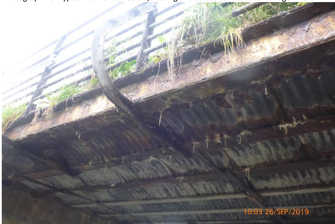
Photograph 11: Typical view of corrosion to outside beams and corrosion to bottom of bracing members.
