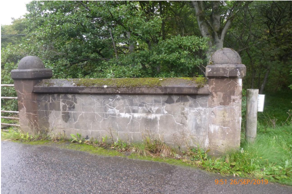
Photograph 35: Typical condition of parapet with cracking and crazing.
