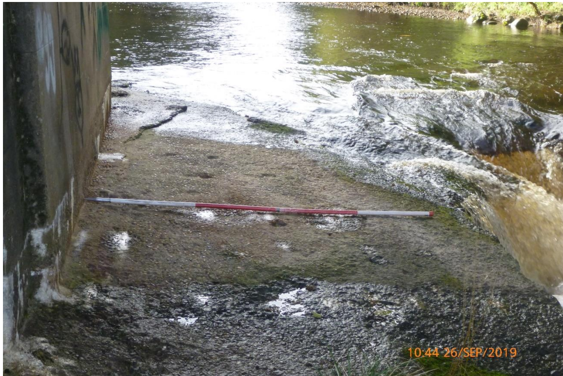
Photograph 26: distance from pier face to scour edge.
