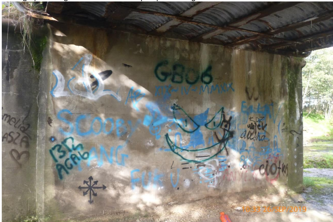
Photograph 17: Example of graffiti present on all abutment and pier faces.
