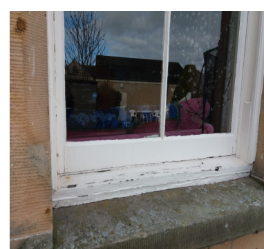
North Elevation bay window, rotten cill, window frame, sash boxes
