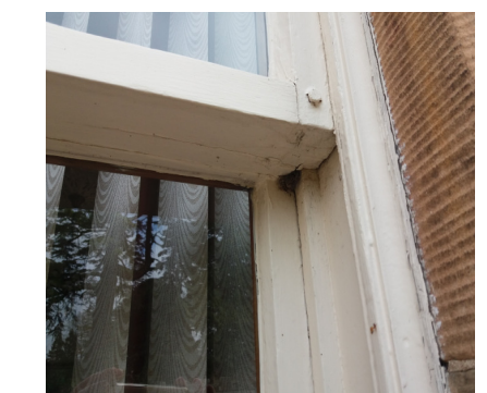
South Elevation bay window, window frames bolted together, joints springing.
