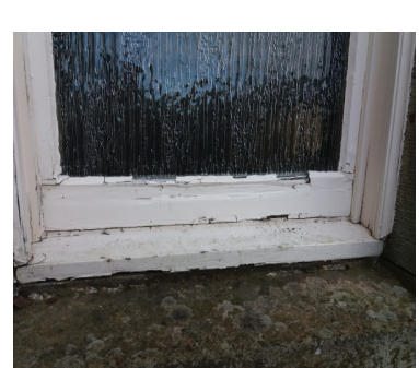
North Elevation Bathroom window, rotten cill, window frame, sash boxes
