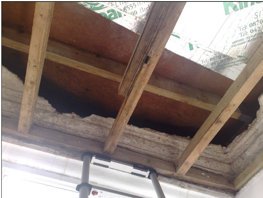
Photo 4 – Same area following removal of the ceiling (was plywood). Note the old plasterwork cornice remains in place. Above the new ceiling structure.
