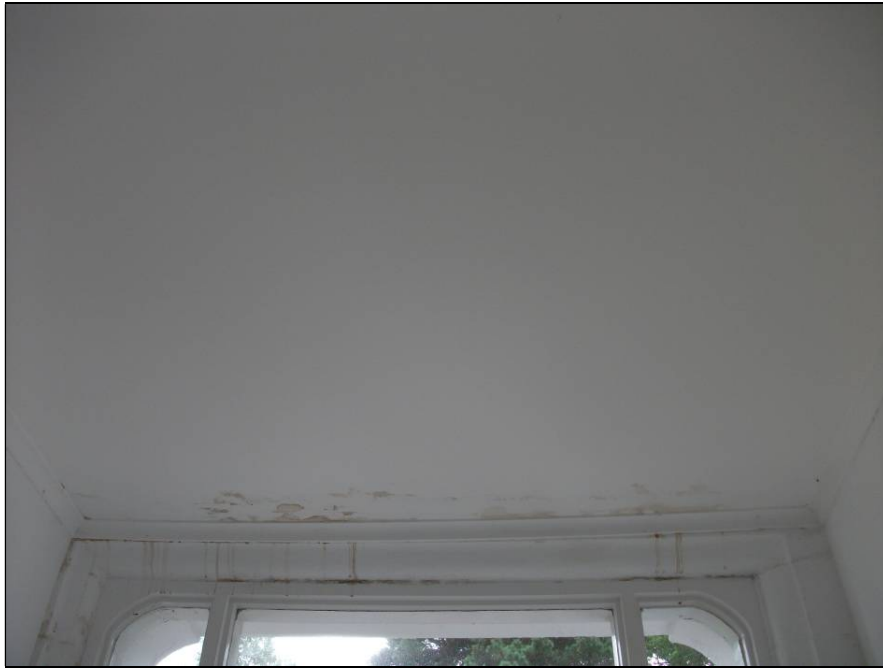
Photo 3 – Ceiling area above the fanlight before ceiling removed. Note the staining of both ceiling and painted stonework.
