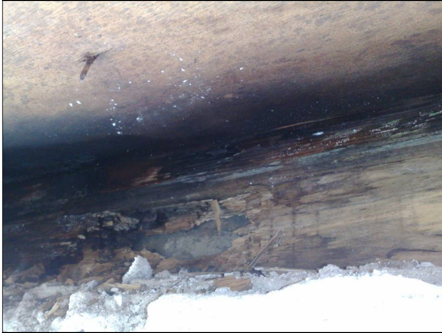
Photo 8 – Roof edge timber element above the front door. Severe timber rot and visibly saturated timber and roof decking. Looks to be an older/original timber left in place when the new roof was fitted.
