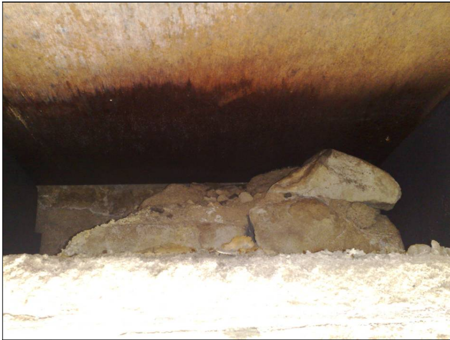
Photo 6 – Another view of the saturated timber decking.
