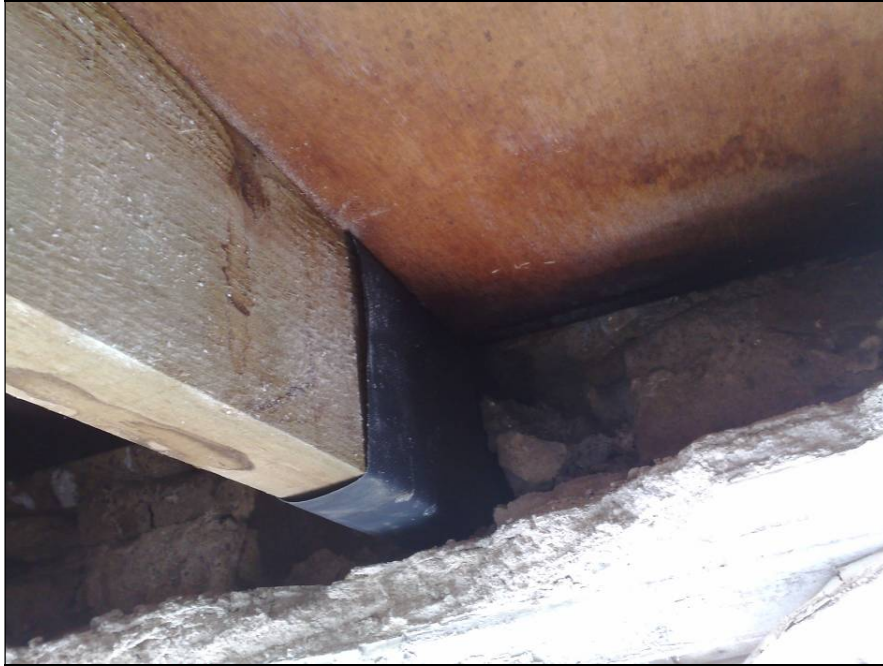
Photo 5 – Shows the replacement roof timbers and roof decking. The dark edge to the decking is very saturated. All the timber showing in this photo had very elevated moisture levels (Protometer used).
