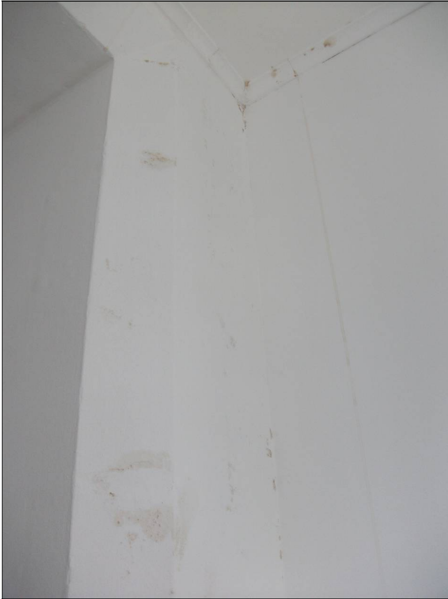
Photo 7 – Interior of the porch. This shows the painted stonework to the right of the inner door(looking from outside), the side wall (plasterboard finish) and part of the ceiling. Note the ceiling and side wall staining and salt damage to the stonework paint finish.
