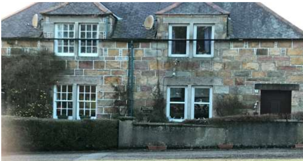
Another example of a property (located in the Square) with UPVC Windows
