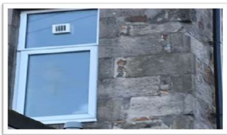
Example of a UPVC window in Hotel 1881 installed prior to current ownership
