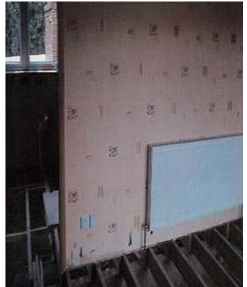
The damage burst pipes can cause
