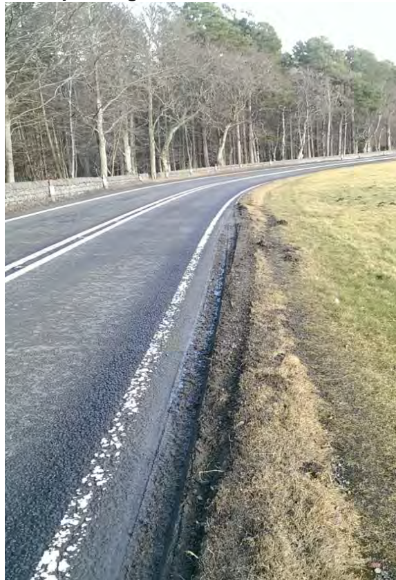
Photograph 3.2 – Example of carriageway over-running on A95
